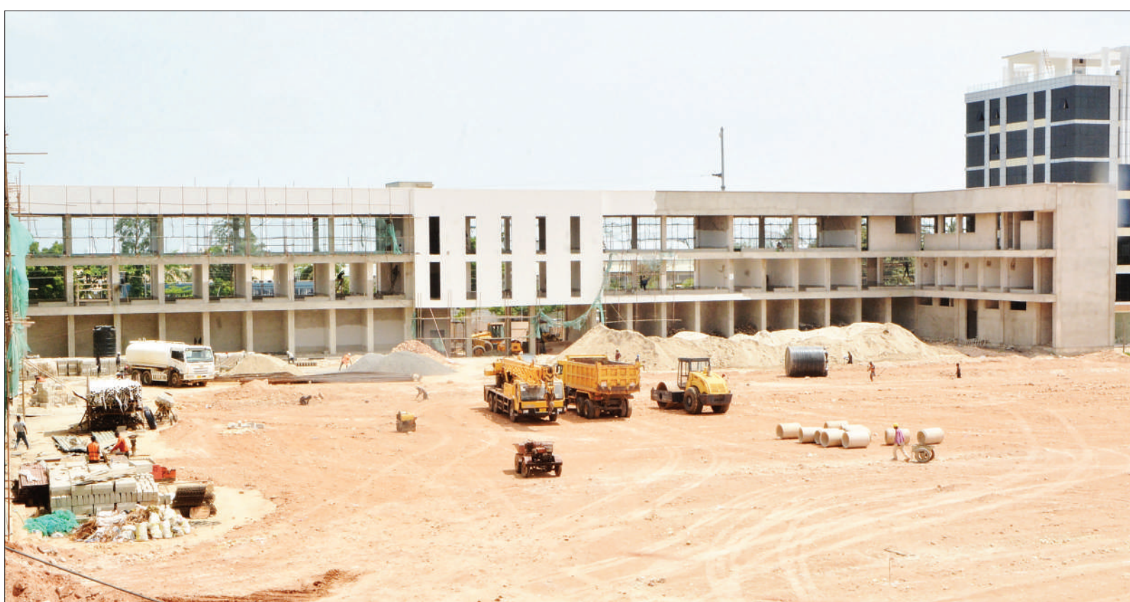
Work on what authorities say will develop into a modern bus stand at Mwanza in Dar es Salaam's Kinondoni municipality has resumed after stopping for quite some time without explanation. Correspondent Miraji Msala captured this scene at the construction site yesterday.
