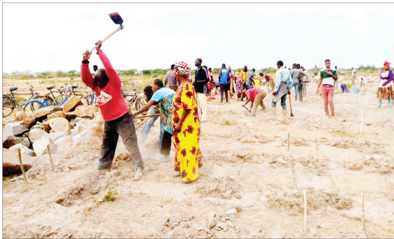
Residents of Nyasaungu village in Ifulifu ward, Musoma Rural constituency, pictured at the weekend busy clearing the site lined up for the construction of Nyasaungu Secondary School's administration building on self-help basis. Photo: Guardian Correspondent
