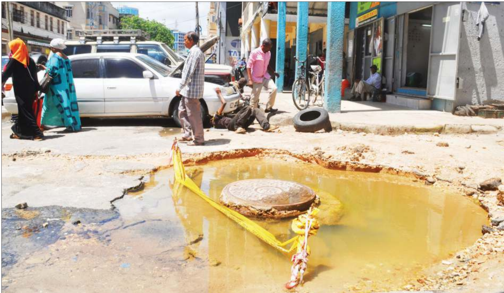
Roads near the Libya Street/Bandi Street intersection in downtown Dar es Salaam rendered impassable to vehicular traffic as the damaged section around the manhole lies unrepaired. Our roving camera captured the scene yesterday. Photo: John Badi
