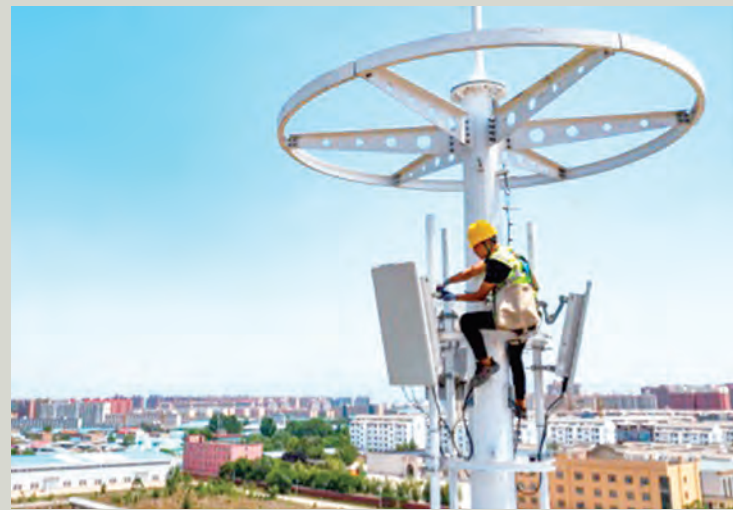
A technician installs equipment at a 5G base station in Yuncheng, north China's Shanxi province, May 17, 2022. File photo
