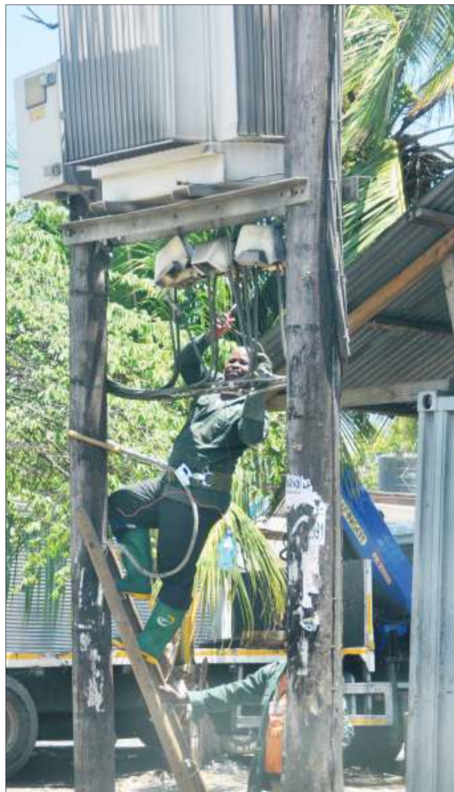
A Tanzania Electric Supply Company (Tanesco) technician repairs a transformer at Mwananyamala kwa Mama Zakaria in Dar es Salaam on Thursday. Photo: John Badi
