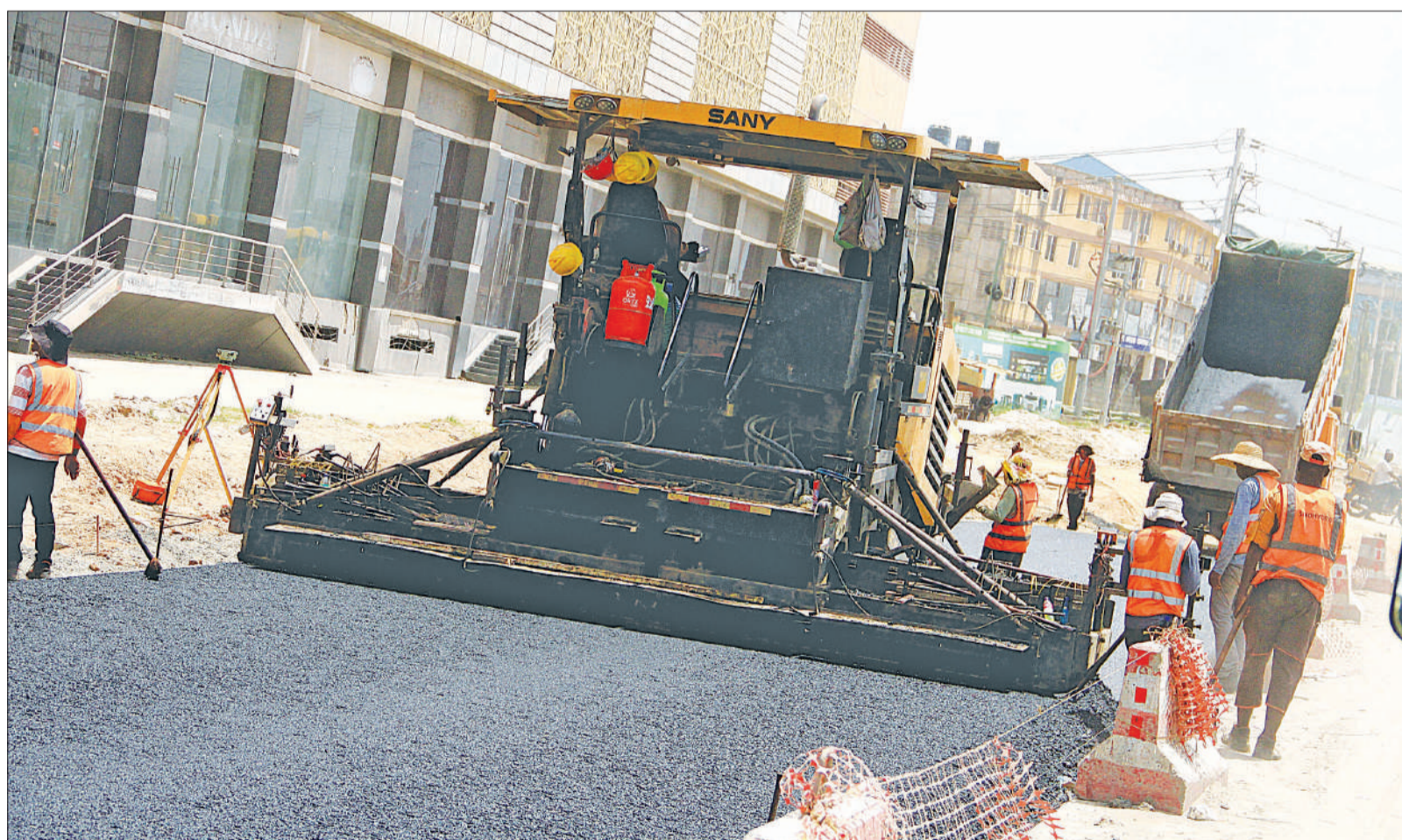
Rehabilitation of Kamata section of Dar es Salaam's Nyerere Road in progress yesterday. Photo: Correspondent Jumane Juma
